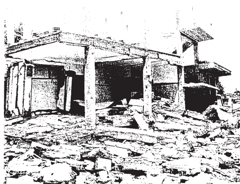
Photo 2 Typical destroyed house located near epicenter at Zemouli city in Algeria.
