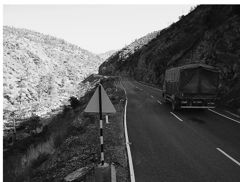
Photo 7 Before situation of slope failure at near Tshozam (Fig. 1⑩). Road shoulders were already depressed due to erosion of valley of Wang Chu (left) and over loading. All of the vehicles were loath to drive at the left side lane. Photo was taken on 1st January, 2010.
