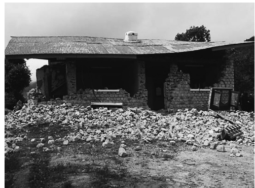
Photo 6 Devastated basic health units (local clinic office). A lot of unframed maisons were collapsed. (Yeshe et al., 2009)
