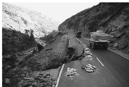
Photo 8 After a month and half of Photo 7. Photo was taken on 14th February, 2010. Left side lane had been absolutely ruined.
