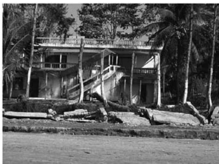
第7図 Damaged building of the resort hotel in the Kuwakata coast
